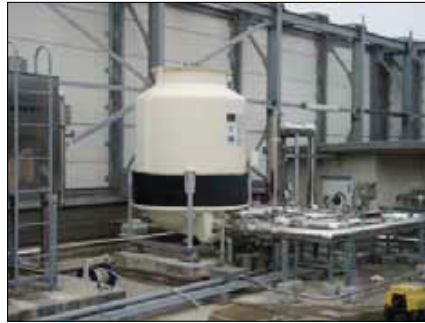
Cooling Tower C
